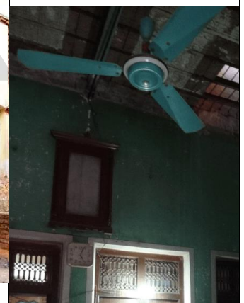
Damaged interior of the old building
